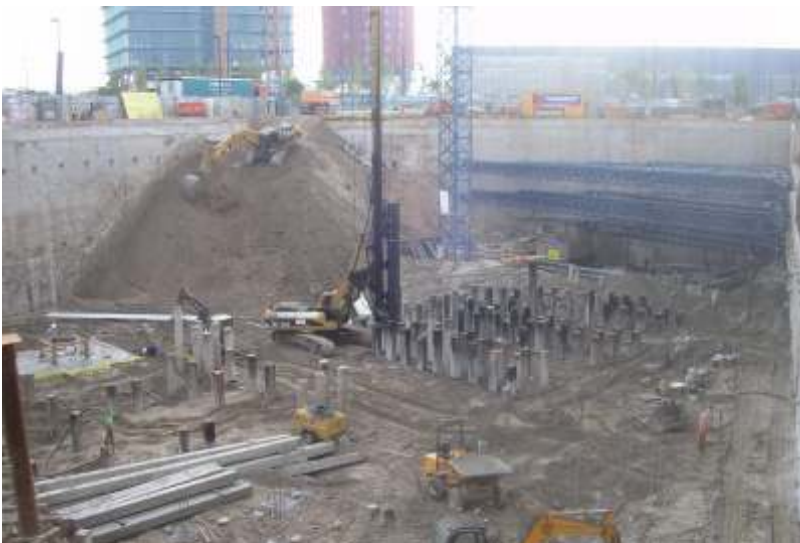
Precast Piling Foundation for Catalonia Hotel at Europa Square, Hospitalet de Llobregat (Barcelona)
