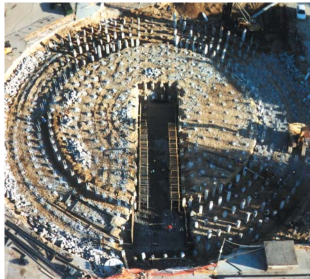
Terra Precastpile foundations for a new 75,000 ton useful load sugar silo in the Plant at Benavente (Zamora)
