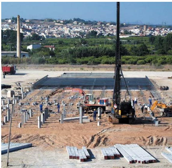
Precast pile foundations and pile trimming for a new coolstore for Hero España. Alcantarilla (Murcia)
