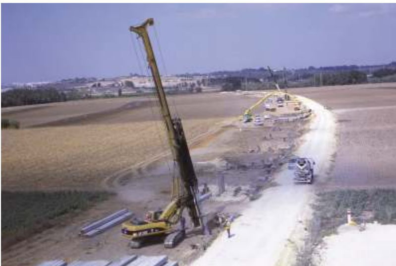
Foundation by Precast Piles for Railway Sevilla-Cadiz. Tranche: Jerez de la Frontera-Cadiz Airport. Subtrante El Portal (Cadiz)
