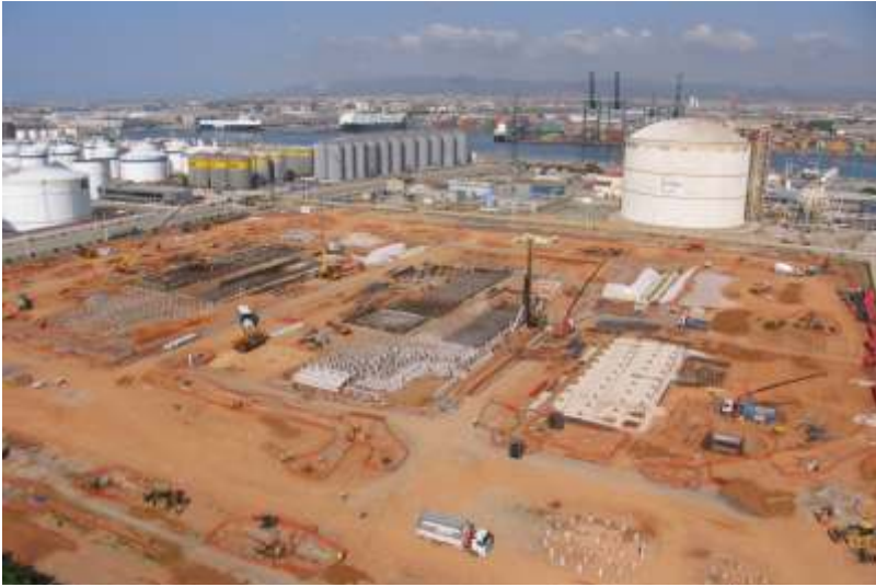
Precast and Prestressed Piling Foundation works for a Combined Cycle Power Plant at Barcelona Seaport
